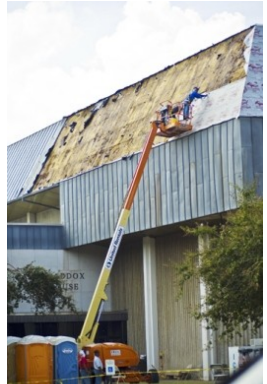
LSU's Carl Maddox Fieldhouse suffered damage to its roof and exterior facade
